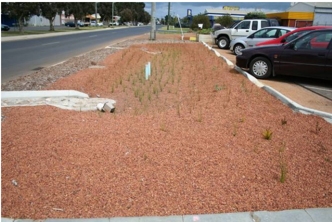
Figure 6. Bioretention system installed to treat carpark runoff in the Busselton Light Industrial Area. (Photograph: Department of Water 2008.)
