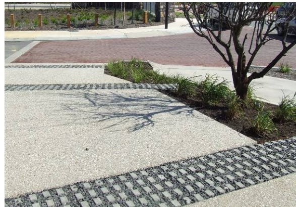
Figure 5. Pervious paving driveway at an urban development in Baldivis. (Photograph: Department of Water 2008.)
